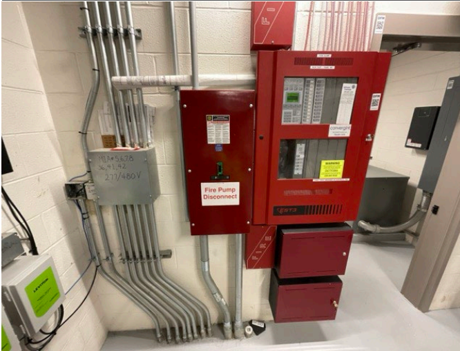
19 - FIRE ALARM PANEL
